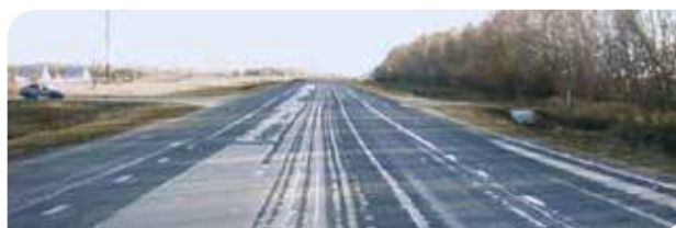
Loss of cover aggregate due to poor adhesion.
